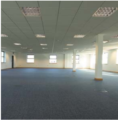
Suspended ceilings with recessed lighting.
