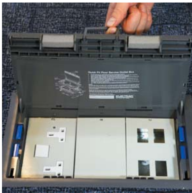
Fully accessed raised floors.
