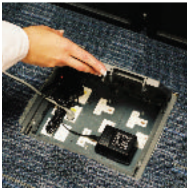
Fully raised access floors.
