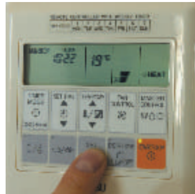
Air conditioning an optional extra (comfort cooling/conditioning).
